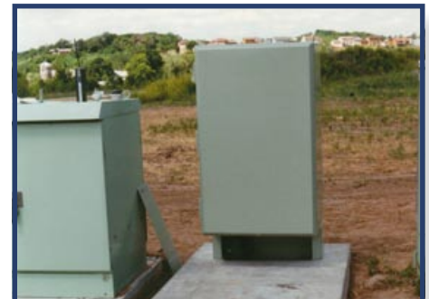
TELECOMMUNICATION CABINET BASE
