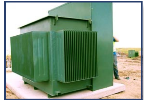
THREE PHASE TRANSFORMER BASE
