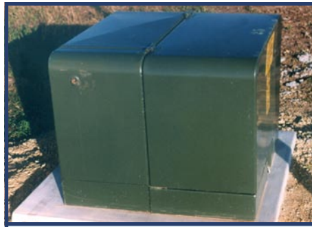
SINGLE PHASE TRANSFORMER BASE
