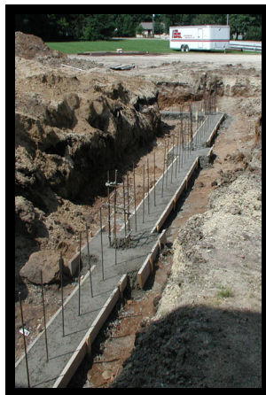
Picture shows the footings, one of the first steps in the new addition.
