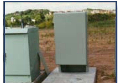
TELECOMMUNICATION CABINET BASE
