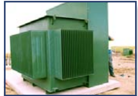
THREE PHASE TRANSFORMER BASE
