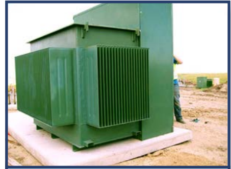
THREE PHASE TRANSFORMER BASE
